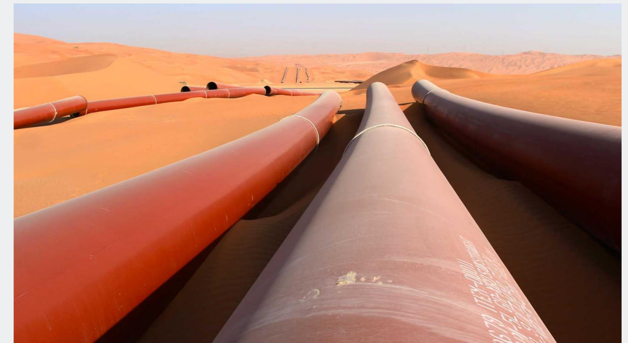
Mster Gas System Expansion -KSA
